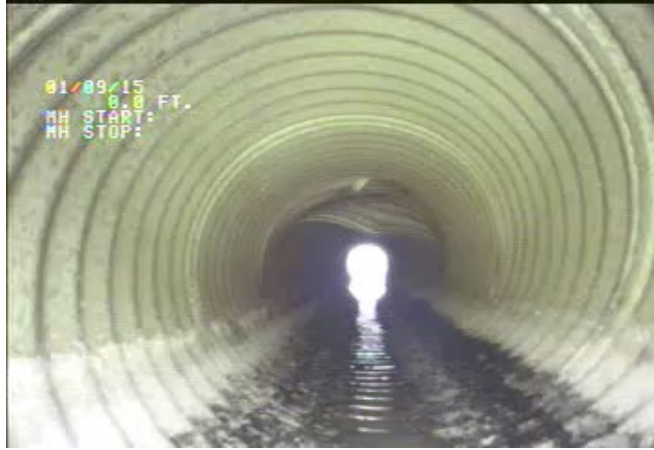
Figure 6. Pre-Rehabilitation – Arizona Crossing - Severe Pipe Deformation
